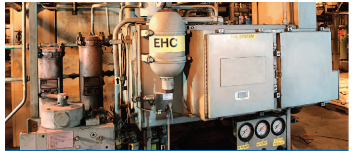
Gas turbines, designed to supply power during periods of peak demand, require fast start up without problems
